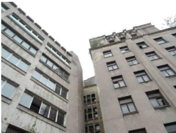
Current buildings - facade of Unit A, Unit B Calea Victoriei no. 216 and no. 218 District 1, Bucharest
